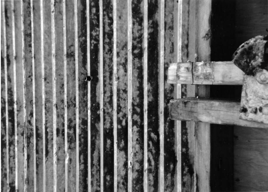
Figure 7-1. Mottled concrete due to moisture locked in by ABS forming
