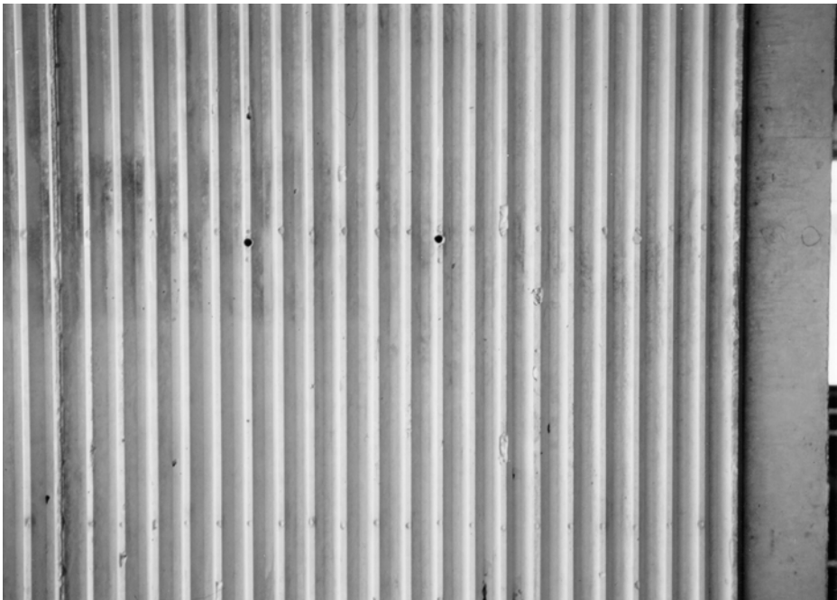
Figure 7-2. Mottled surface has lightened after period of drying
