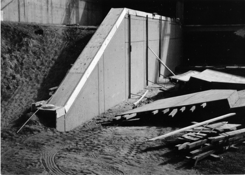
Figure 7-3. Protection of architectural concrete
