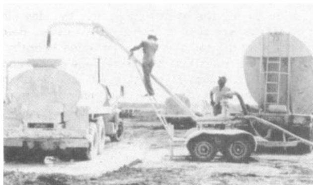
Figure 4-30. Jet slurry mixing plant.
