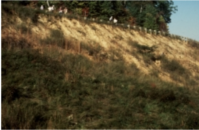
Figure 18-1a Eroding fill slope
