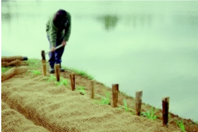
Figure 16-55a Installing dead stout stakes in reed clump system (Robbin B. Sotir & Associates photo)
