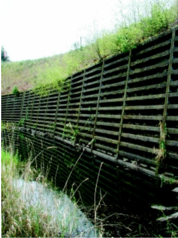
a. Manufactured Retention System. Salmon Creek, Tributary to Columbia River. 2002.
