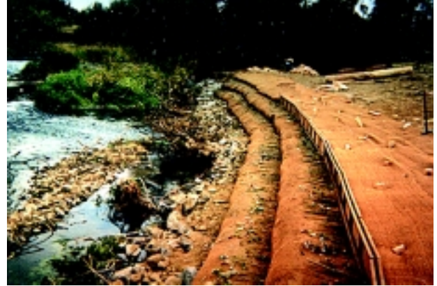
c. Large Woody Debris embedded in Rock Toe. Salmon Creek, Tributary to Columbia River. Source: Inter-Fluve, Inc.
