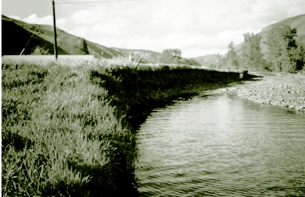
Figure 5-10. Left-bank erosion on the Tucannon River.
