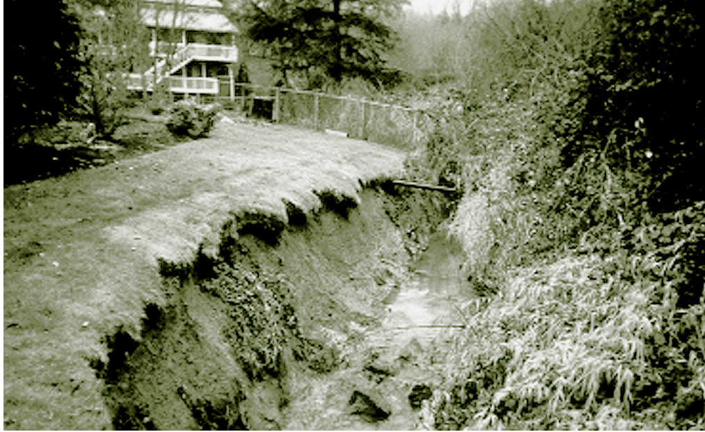
Figure F-5. Channel Degradation. An example of channel instability in a degrading channel.
