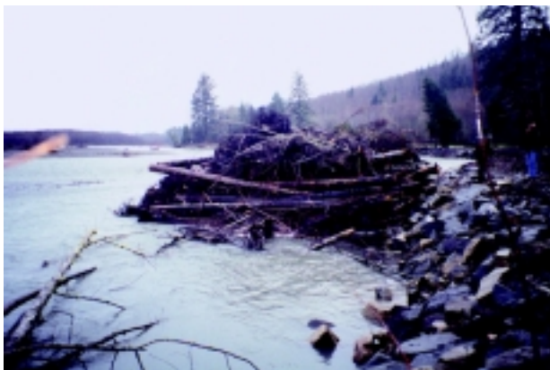
b. Large Woody Debris embedded and collected on Groin. Hoh River. 1998.
