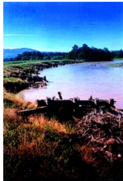
f. Wood Groins. Nooksack River. 1998.
