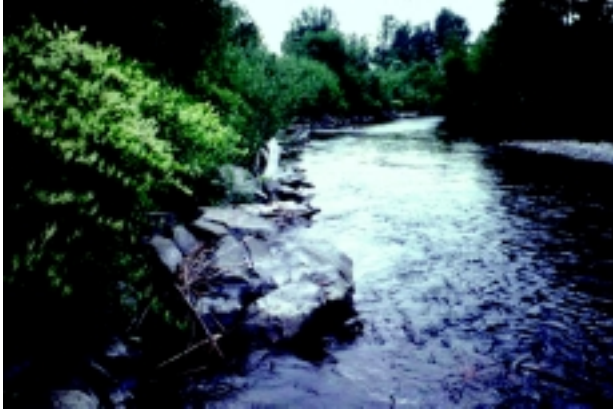
a. Roughened-Rock Toe with reinforced large woody debris and plantings. Cedar River. 1999.
