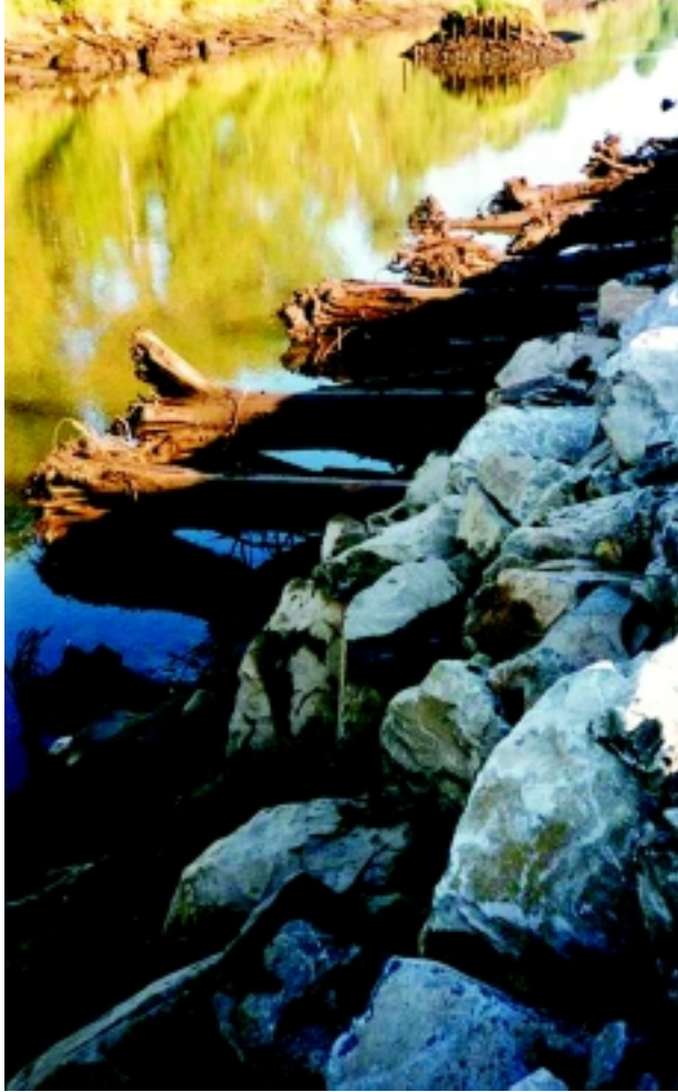
a. Large Woody Debris embedded in Rock Toe. Green River. Source: King County Department of Natural Resources.
