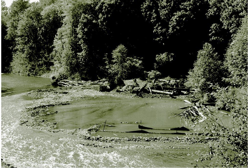
Figure M-2. Partial isolation minimizes the continued release of sediments when working in a wet-channel environment.
