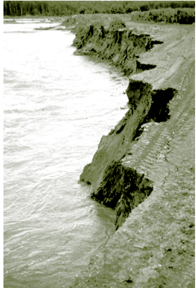
Figure 5-5. Ground view of erosion on the Nooksack River.
