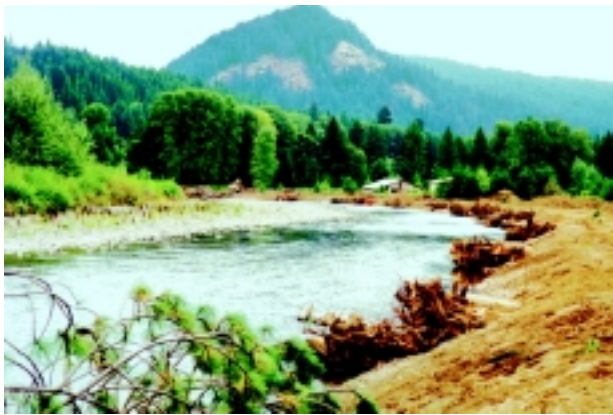
a. Wood Groins with bank reshaping and plantings. During Construction. Wind River. 1999.
