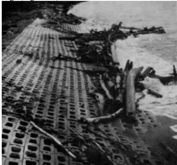
Figure 49 Control Block Revetment
