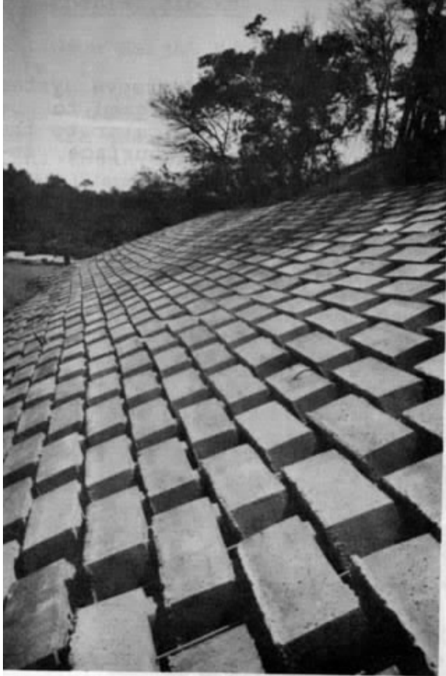
Figure 53 Terrafix Block Revetment
