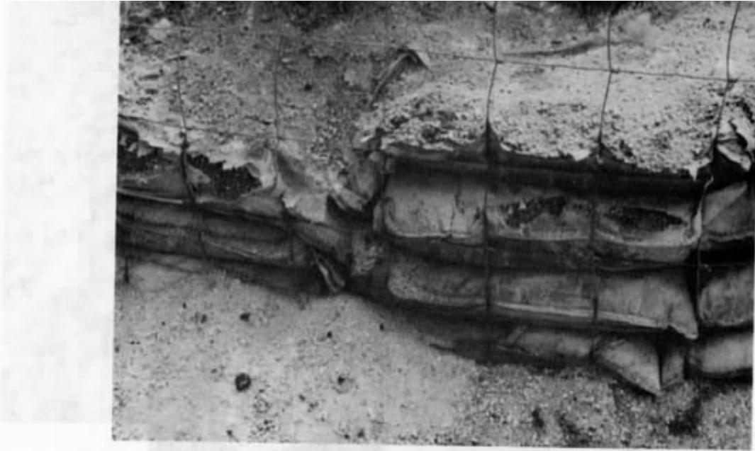
Figure 56 Deterioration of Sand Bags Under Ultraviolet Light
