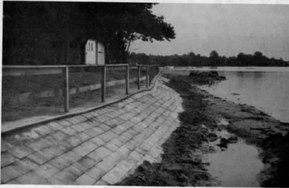
Figure 50 Shiplap Block Revetment
