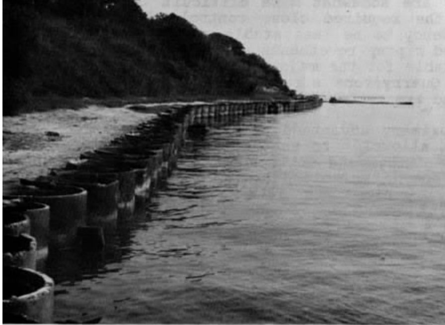
Figure 41 Used Concrete Pipe Bulkhead
