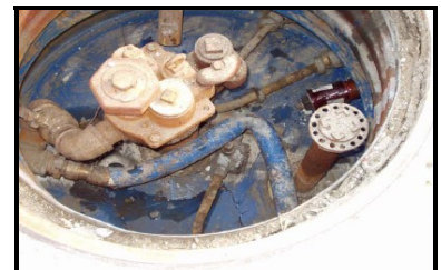
Flexible piping is kinked
