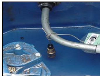
Liquid sump sensor
