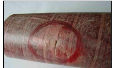
Fiberglass piping is cracked
