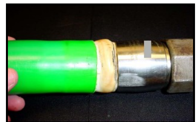
Flexible piping is bulging
