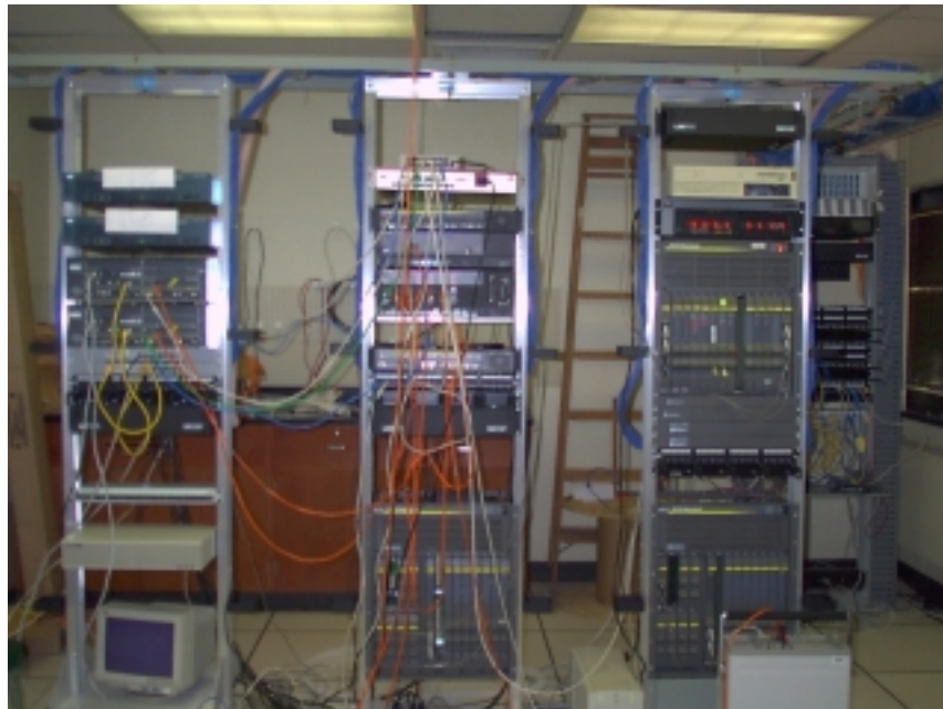
Figure 23. Center for Telecommunications Education and Research Lab (CTER)
