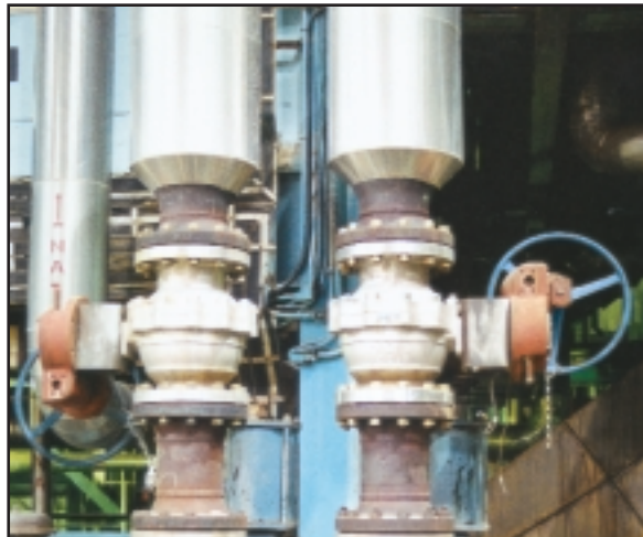
8" Hot caustic isolation valves at 345°F.
