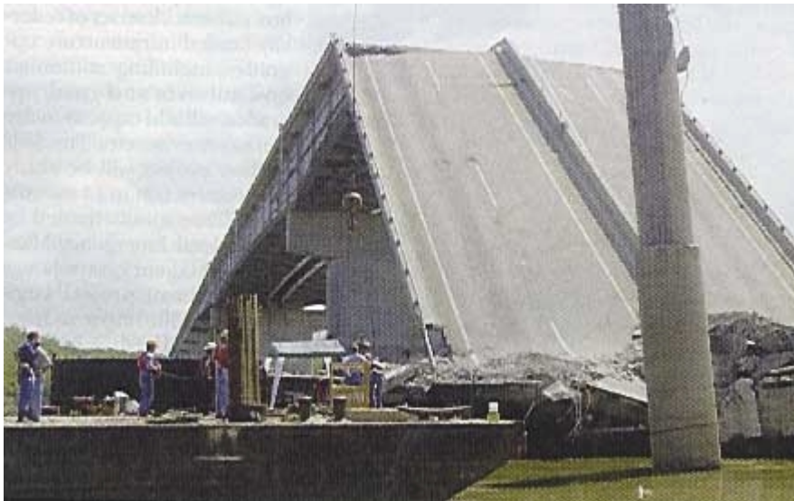
Figure 8: The barge in the foreground shattered bridge piers causing a section of the interstate highway to tilt into the river.
