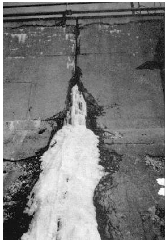
Figure 2-28. Water seepage through joint
