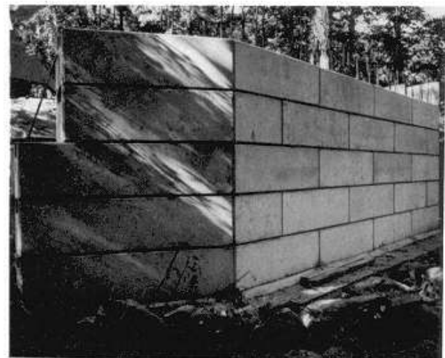
Figure 8-52. Front view of precast abutment prior to placing concrete cap, Ulsterville Bridge
