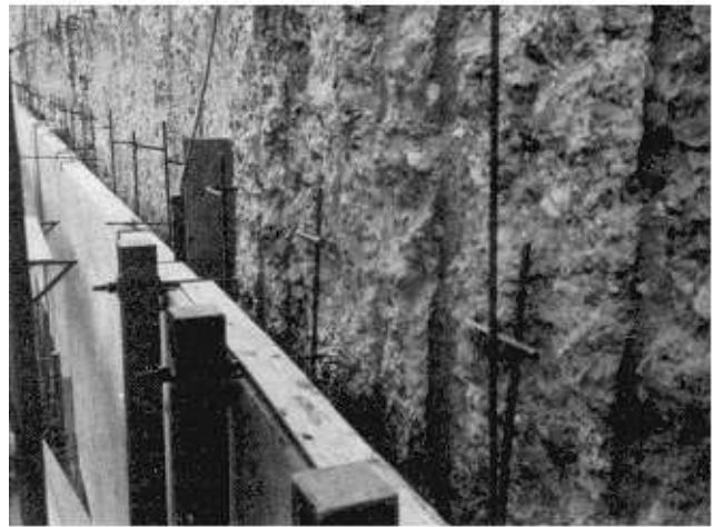
Figure 8-15. Installation of precast concrete stay-in-place forms at Troy Lock, Hudson River (Miles 1993)
