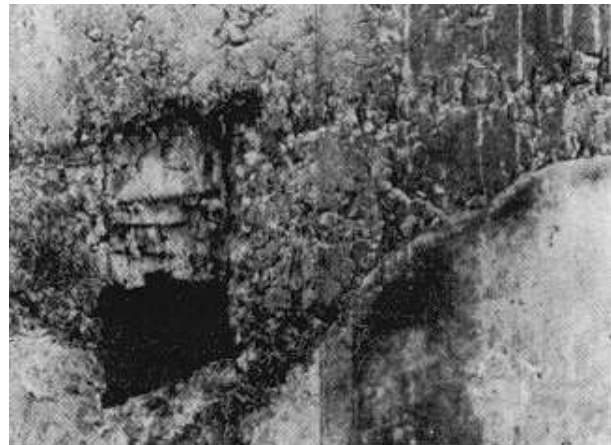
Figure 2-2. Honeycombing and cold joint
