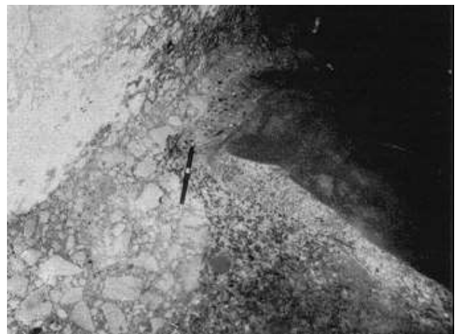
Figure 2-20. Smooth, worn, abraded concrete surface caused by abrasion of waterborne debris
