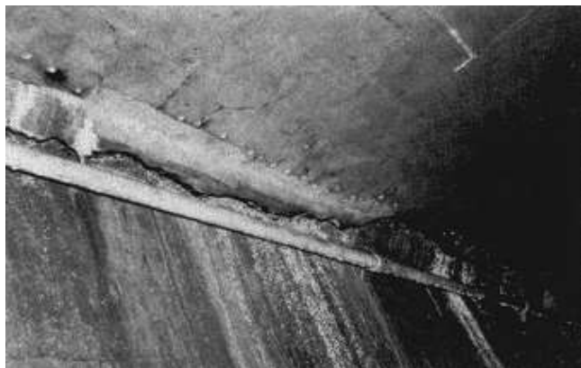
Figure 2-11. Isolated crack caused by structural overload
