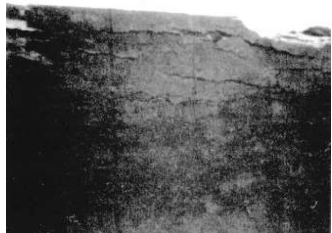
Figure 2-10. Parallel individual cracking caused by freezing and thawing
