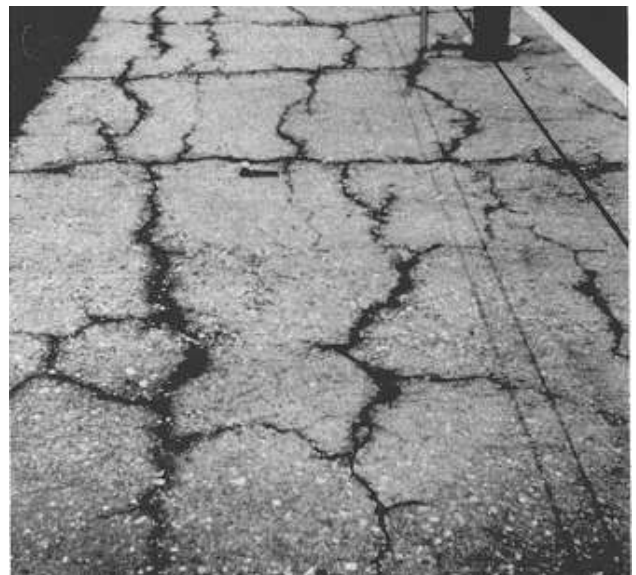
Figure 2-6. Pattern cracking resulting from alkali-silice reaction
