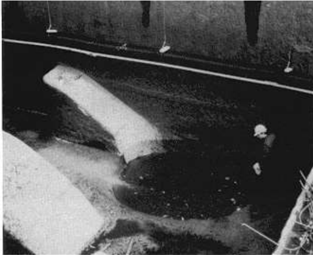
a. Scour holes behind baffles
