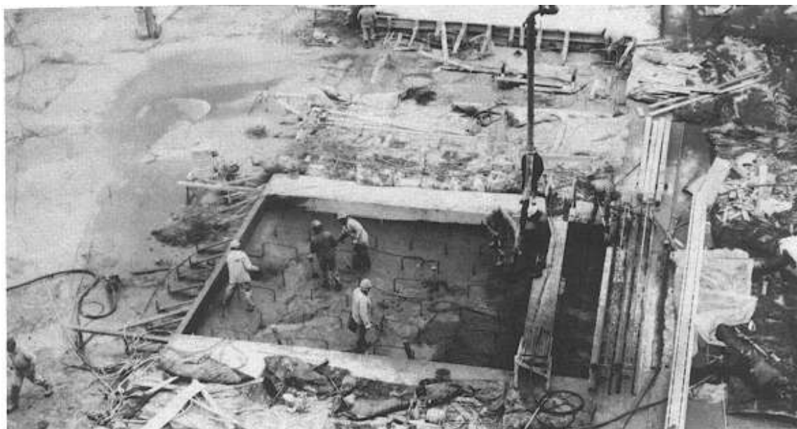
Figure 8-36. Pumping silica-fume concrete into the stilling basin from the top of the right training wall, Kinzua Dam
