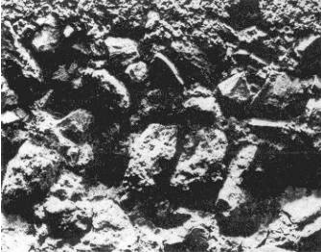
Figure 2-21. Rough, pitted concrete surface caused by cavitation
