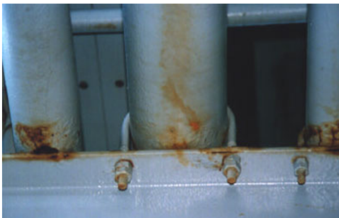
Source: Deepwater Corrosion Services, Inc.
