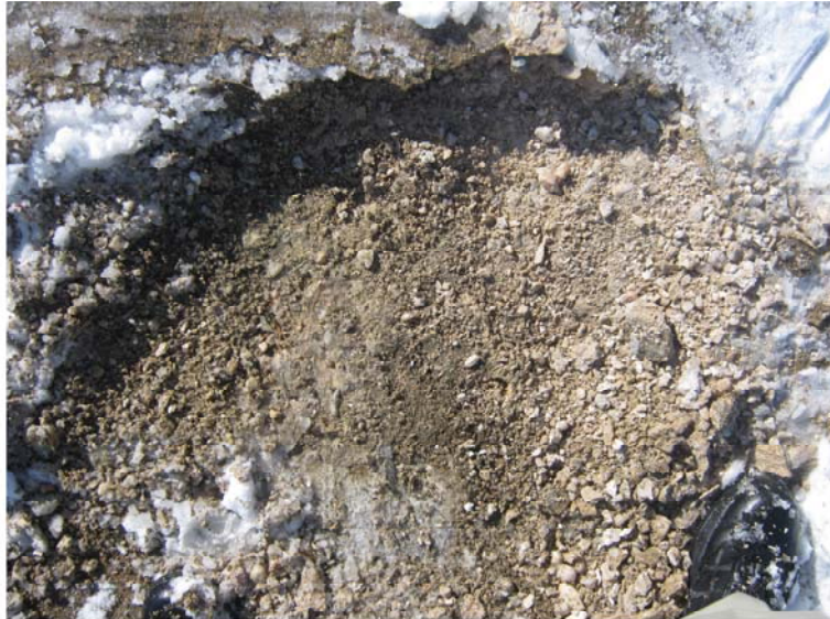
Freeze-Thaw Damage of a Dome Slab
