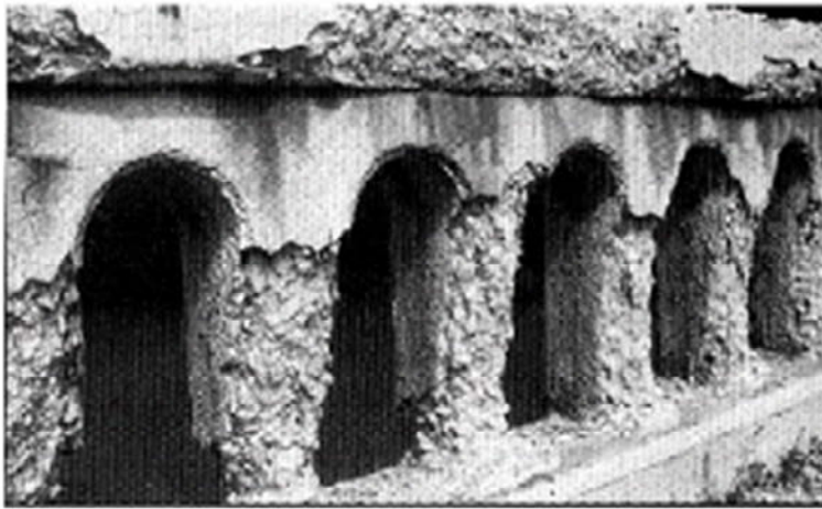
Typical Example of Non-Air-Entrained Concrete Deteriorated from Freeze-Thaw Action
