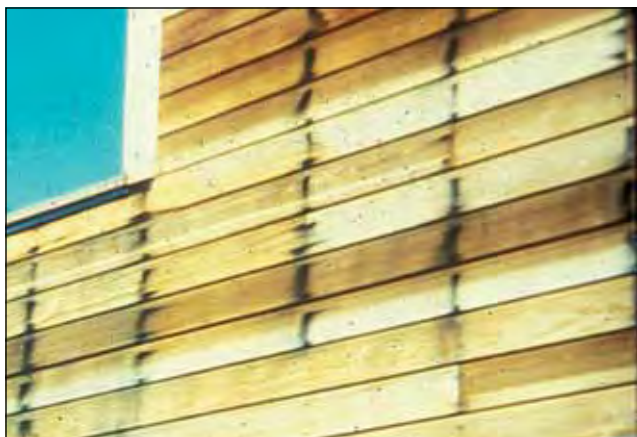
Figure 16-28. Iron stain on newly installed wood siding. Poor quality galvanized nails corrode easily and, like uncoated steel nails, usually cause unsightly staining of the wood.
