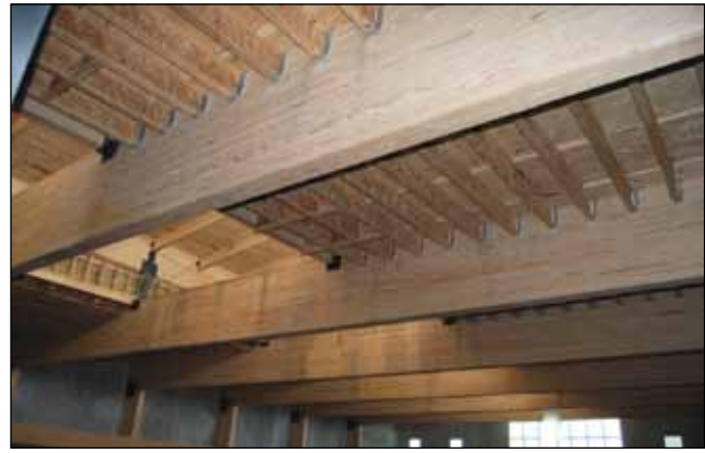
Figure 11–1. Wood-based composites used in the new Centennial Research Facility at the Forest Products Laboratory. Glulam timbers support composite I-joists and plywood sheathing. (Photo by Steve Schmieding, Forest Products Laboratory.)
