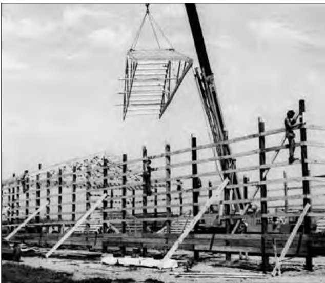
Figure 6–6. Poles provide economical foundation and wall systems for agricultural and storage buildings.
