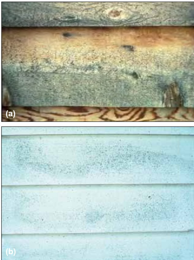
Figure 16–24. Mildew is most common in shaded, moist, or protected areas (a) on wood and (b) on painted wood.
