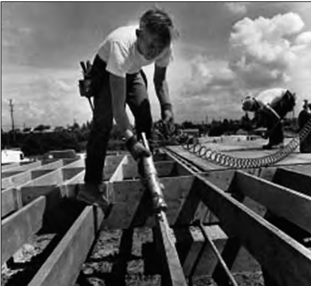
Figure 10–7. A pressurized extruder applies a single bead of elastomeric construction adhesive to floor joists for assembly of a plywood floor system.
