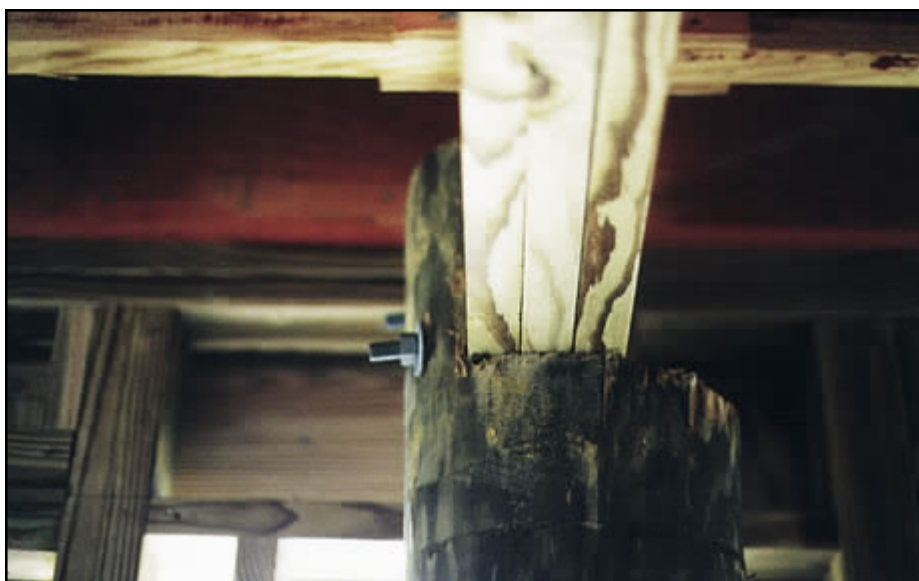
Figure 13-3 Overnotched pile. Also note mislocated bolt.
