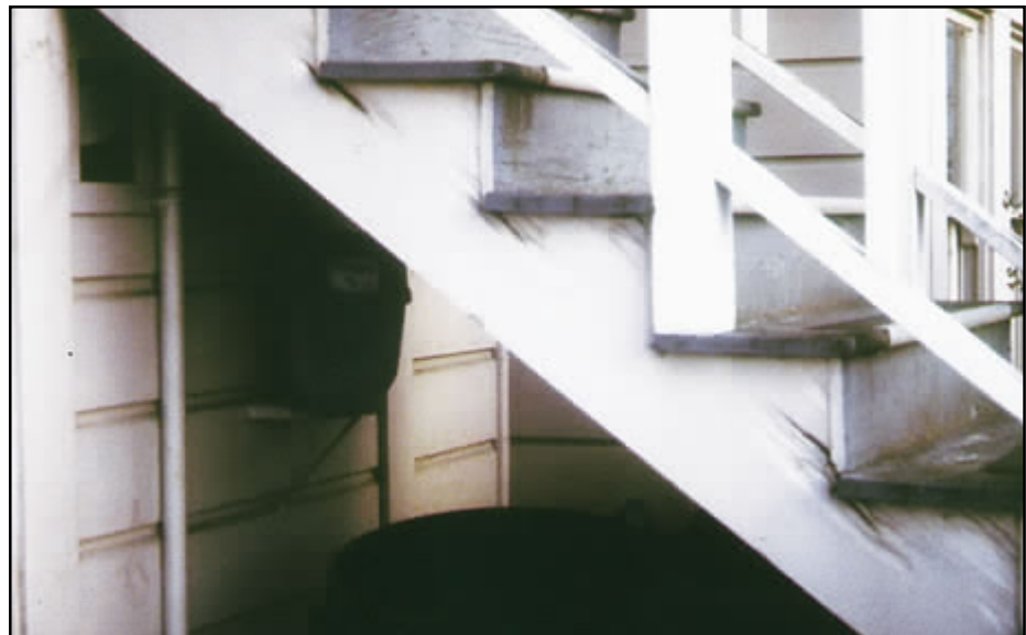
Figure 13-17 Deterioration in a notched stair stringer.
