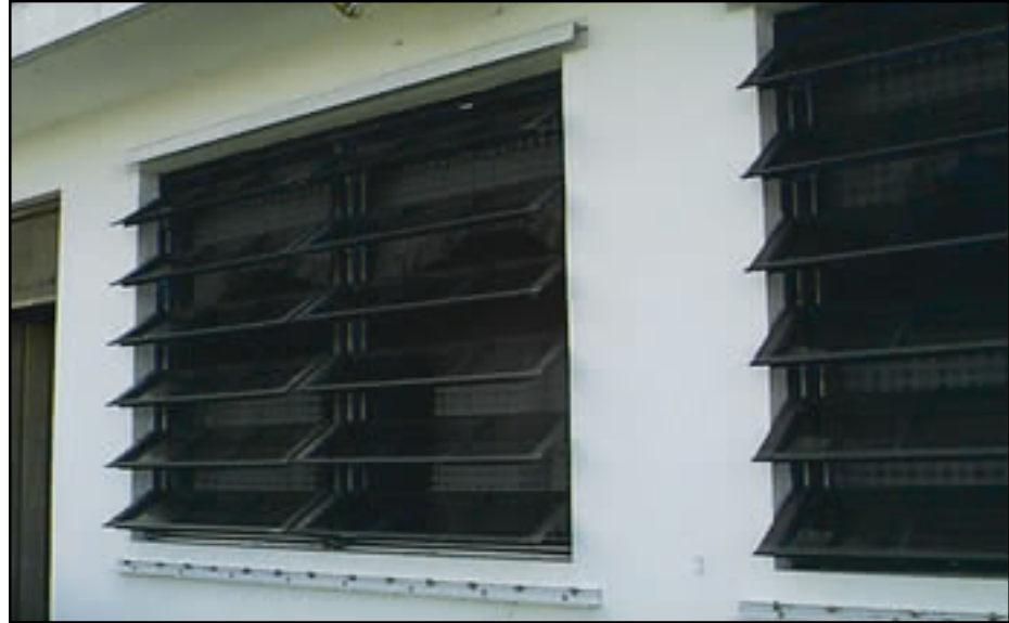
Figure 12-96 Hurricane Georges (1998), Puerto Rico. Permanently installed shutter tracks.
