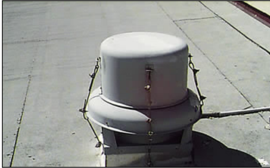
Figure 12-113 Typhoon Paka (1997), Guam. Stainless steel cables for strengthening fan cowlings and vent hoods.
