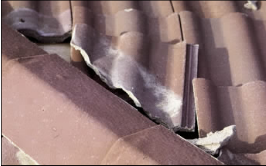
Figure 12-105 Northridge Earthquake, California. The tile in the center of this photograph slipped out from underneath the hip tiles. The tile that slipped was trimmed to fit at the hip. The trimming eliminated the nail holes and no other attachment was provided. The friction fit was inadequate to resist the seismic forces.
