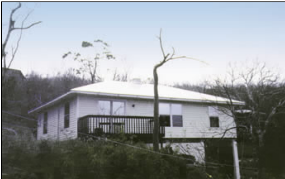
Figure 12-30 Hurricane Marilyn (1995), U.S. Virgin Islands. Hip roof that survived high winds with little to no damage.
