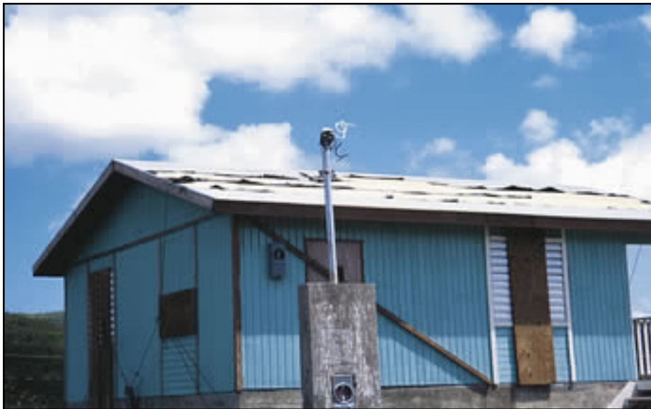
Figure 12-119 Hurricane Georges (1998), Puerto Rico. Concrete pylon used for overhead service mast.
