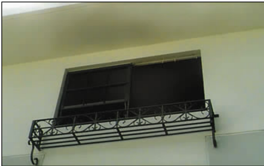
Figure 12-92 Hurricane Georges (1998), Puerto Rico. Inadequate window frame attachment caused the window frame to be pulled out of the wall.
