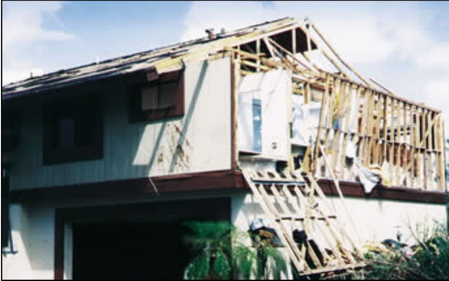
Figure 12-4 Hurricane Andrew (1992), Dade County, Florida. Second-story wood framing (on first-story masonry). End gable and wall failure.
