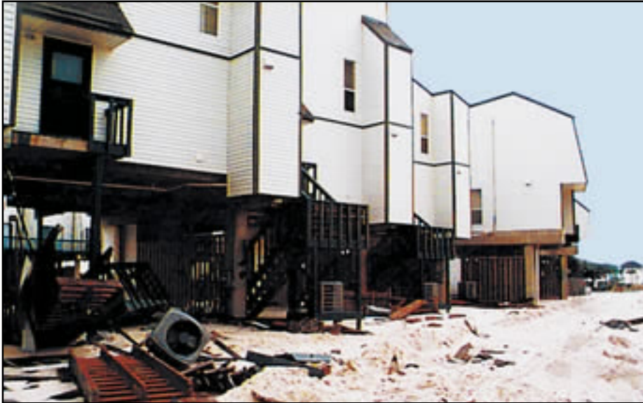
Figure 12-114 Hurricane Georges (1998), U.S. Gulf Coast. Mechanical equipment damaged as a result of insufficient elevation.
