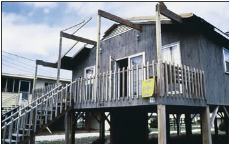
Figure 12-5 Hurricane Diana (1984). Uplift failure of a porch roof.
