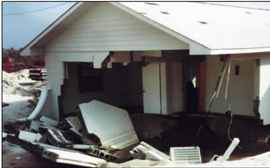
Figure 12-11 Hurricane Fran (1996), North Carolina. Failure of a coastal A-zone building constructed on a masonry wall and slab-on-grade foundation. The failure resulted from undermining of the foundation by severe scour.
