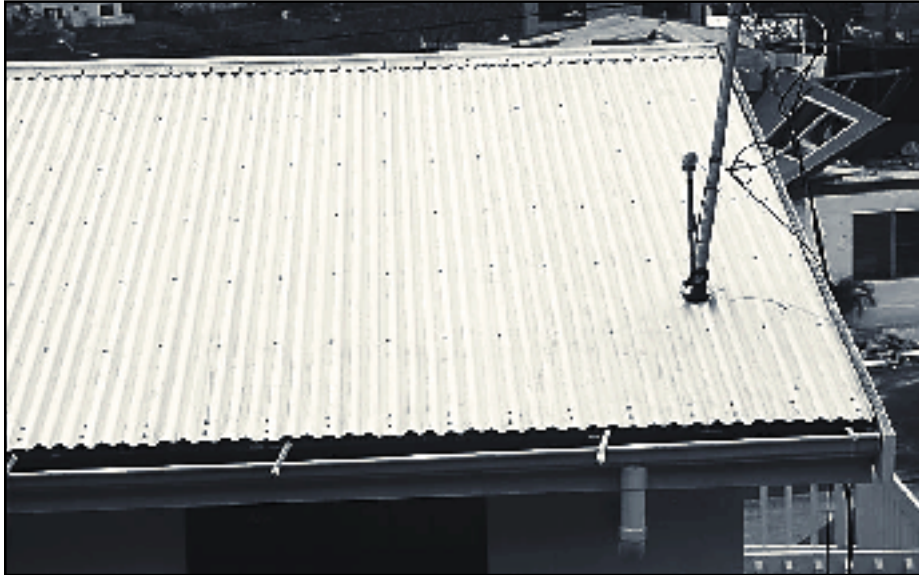
Figure 12-118 Hurricane Marilyn (1995), U.S. Virgin Islands. Damage caused by dropped overhead service.
