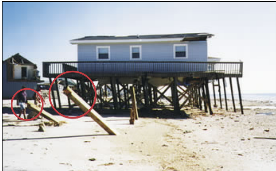
Figure 12-12 Hurricane Fran (1996), North Carolina. Building pilings (circled) snapped at top.
