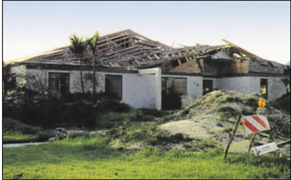
Figure 12-62 Hurricane Andrew (1992), Dade County, Florida. Gable- end failure.
