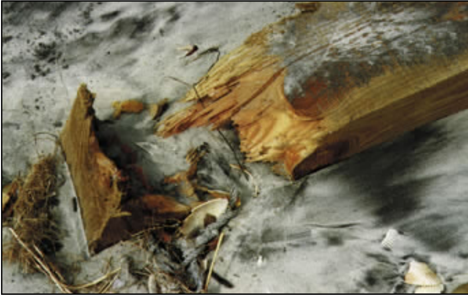
Figure 12-79 Hurricane Fran (1996), North Carolina. Square wood pile failure at edge knot.
