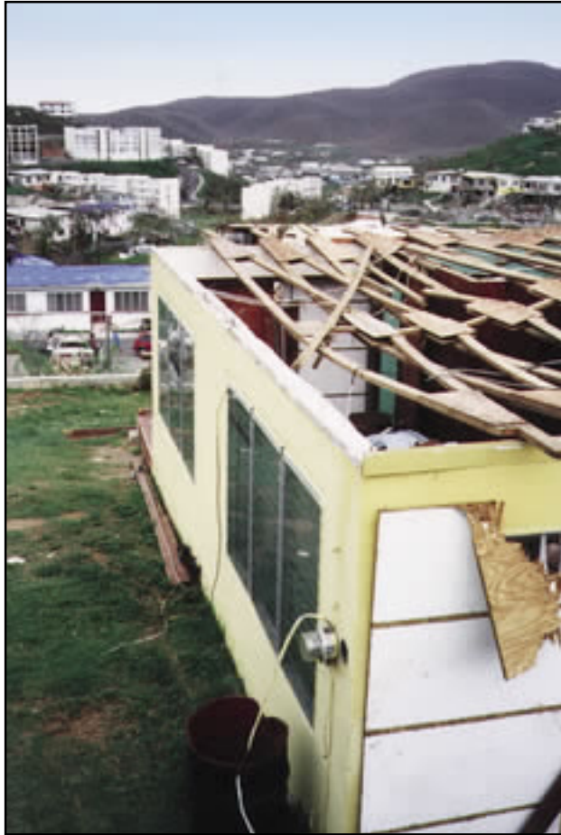
Figure 12-29 Hurricane Marilyn (1995), U.S. Virgin Islands. Gable-end failure caused by high winds.
