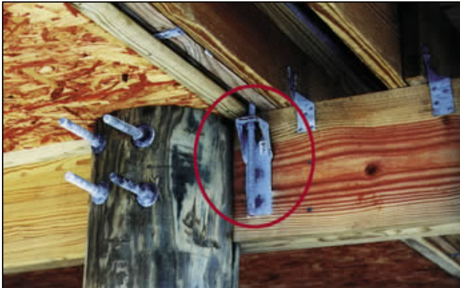
Figure 12-46 Shearwall holddown connector with bracket attached to a wood beam.
