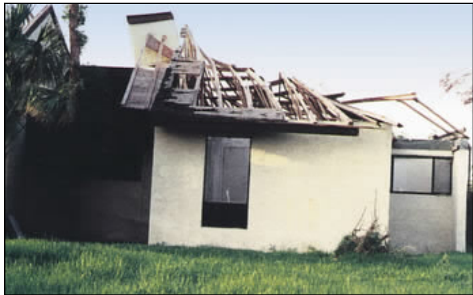
Figure 12-3 Hurricane Andrew (1992), Dade County, Florida. Roof structure failure due to inadequate bracing.
